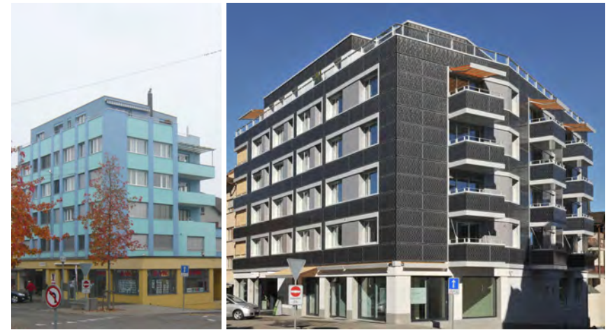
Romanshorn: Plus energy renovation with PV-facade – built 1961 / renovation 2012 Norman Foster Solar Award 2013 and European Solar Price 2013
